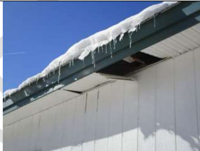
Location: 347 Depot St Jamaica, VT Photo Taken By: Richard Lalancette, P.E. IMG: 136 Description: Soffit repair needed
