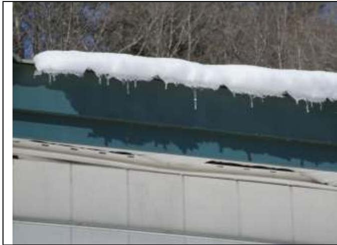
Location: 347 Depot St Jamaica, VT Photo Taken By: Richard Lalancette, P.E. IMG: 137 Description: Soffit repair needed
