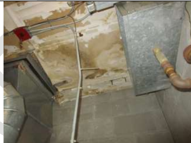
Location: 347 Depot St Jamaica, VT Photo Taken By: Richard Lalancette, P.E. IMG: 197 Description: Deteriorated ceiling in new furnace room
