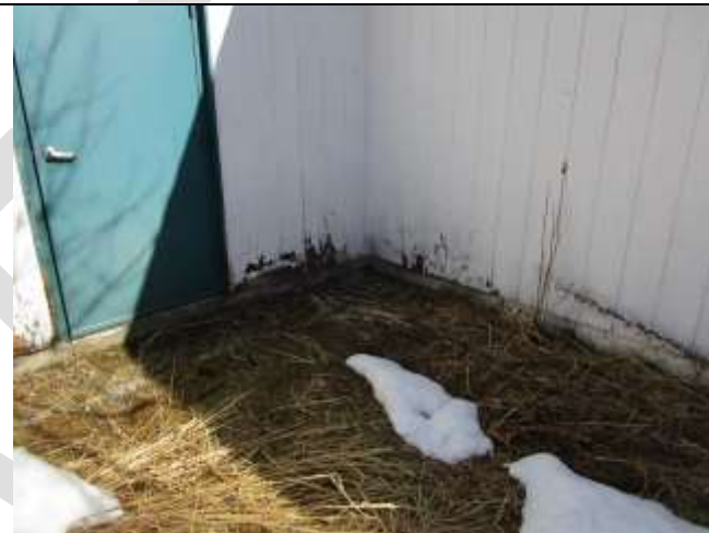
Location: 347 Depot St Jamaica, VT Photo Taken By: Richard Lalancette, P.E. IMG: 161 Description: Rot in lower siding at rear of building
