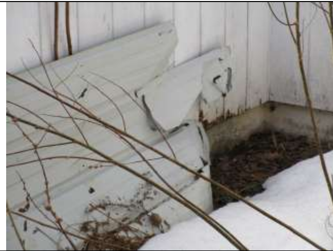
Location: 347 Depot St Jamaica, VT Photo Taken By: Richard Lalancette, P.E. IMG: 159 Description: Rot in lower siding at rear of building
