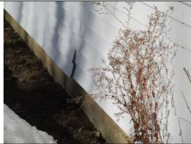
Location: 347 Depot St Jamaica, VT Photo Taken By: Richard Lalancette, P.E. IMG: 147 Description: Loose siding at left side of building
