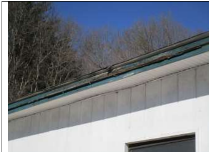
Location: 347 Depot St Jamaica, VT Photo Taken By: Richard Lalancette, P.E. IMG: 164 Description: Rot in soffit fascia trim
