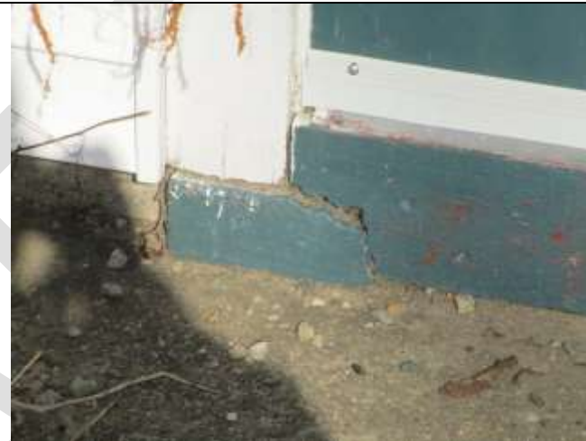
Location: 347 Depot St Jamaica, VT Photo Taken By: Richard Lalancette, P.E. IMG: 145 Description: Damaged door threshold at left front of building
