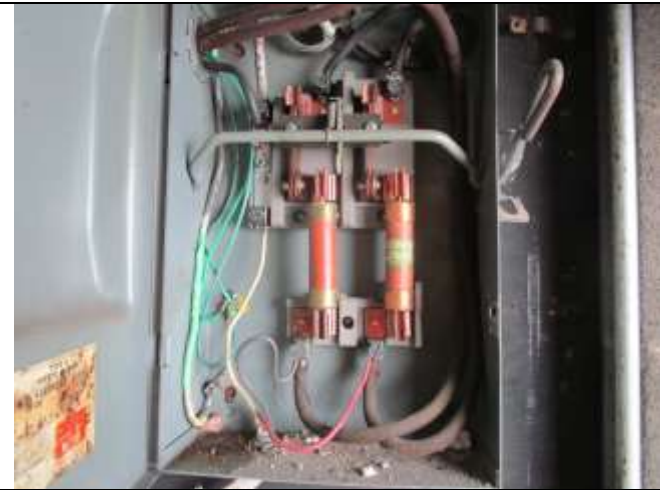
Location: 347 Depot St Jamaica, VT Photo Taken By: Richard Lalancette, P.E. IMG: 191 Description: Fused main switch for original portion of building
