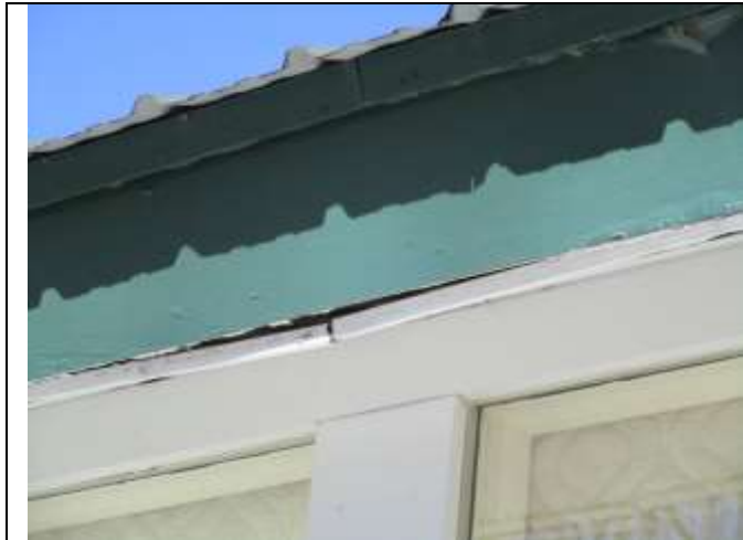
Location: 347 Depot St Jamaica, VT Photo Taken By: Richard Lalancette, P.E. IMG: 148 Description: Loose soffit trim at left side of building
