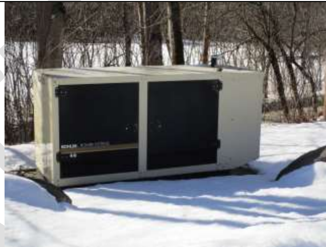
Location: 347 Depot St Jamaica, VT Photo Taken By: Richard Lalancette, P.E. IMG: 119 Description: Generator
