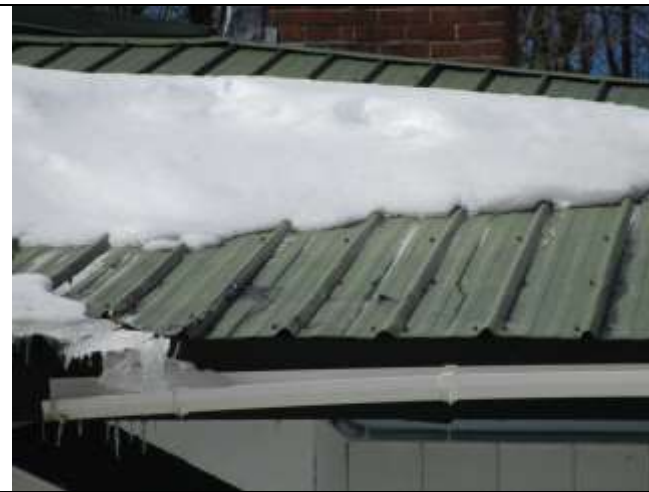
Location: 347 Depot St Jamaica, VT Photo Taken By: Richard Lalancette, P.E. IMG: 175 Description: Damaged roof surface at front entry
