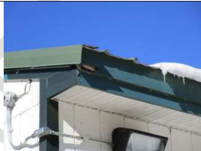
Location: 347 Depot St Jamaica, VT Photo Taken By: Richard Lalancette, P.E. IMG: 141 Description: Rot in soffit fascia trim
