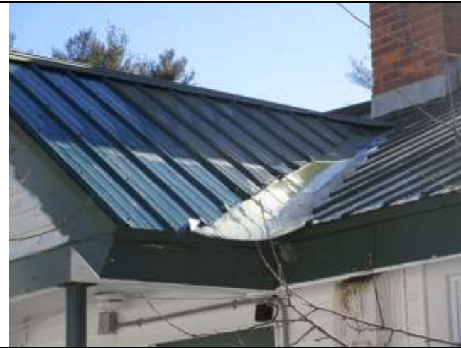
Location: 347 Depot St Jamaica, VT Photo Taken By: Richard Lalancette, P.E. IMG: 179 Description: Damaged roof at rear valley
