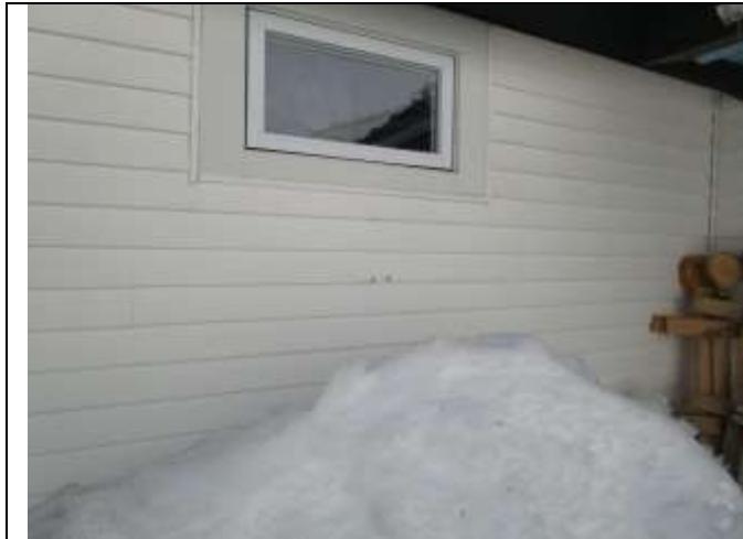
Location: 347 Depot St Jamaica, VT Photo Taken By: Richard Lalancette, P.E. IMG: 144 Description: Damaged vinyl siding
