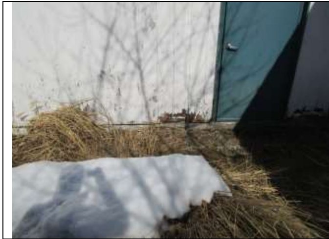
Location: 347 Depot St Jamaica, VT Photo Taken By: Richard Lalancette, P.E. IMG: 162 Description: Rot in lower siding at rear of building
