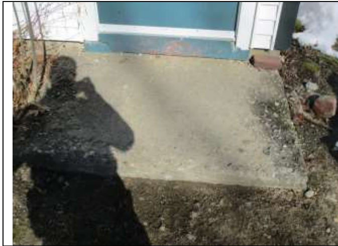
Location: 347 Depot St Jamaica, VT Photo Taken By: Richard Lalancette, P.E. IMG: 146 Description: Deteriorated concrete platform at left front of building
