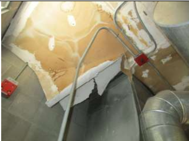
Location: 347 Depot St Jamaica, VT Photo Taken By: Richard Lalancette, P.E. IMG: 196 Description: Deteriorated ceiling in new furnace room
