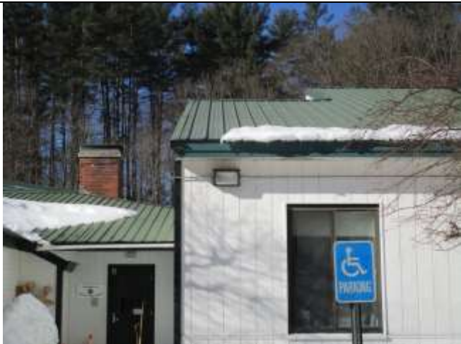
Location: 347 Depot St Jamaica, VT Photo Taken By: Richard Lalancette, P.E. IMG: 131 Description: Typical building mounted lighting
