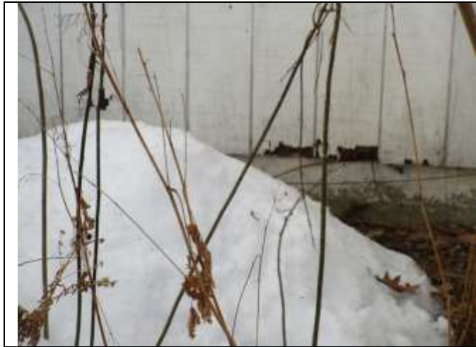
Location: 347 Depot St Jamaica, VT Photo Taken By: Richard Lalancette, P.E. IMG: 158 Description: Rot in lower siding at rear of building
