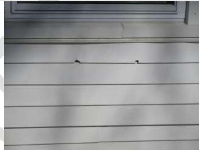
Location: 347 Depot St Jamaica, VT Photo Taken By: Richard Lalancette, P.E. IMG: 149 Description: Damaged siding at left side of building
