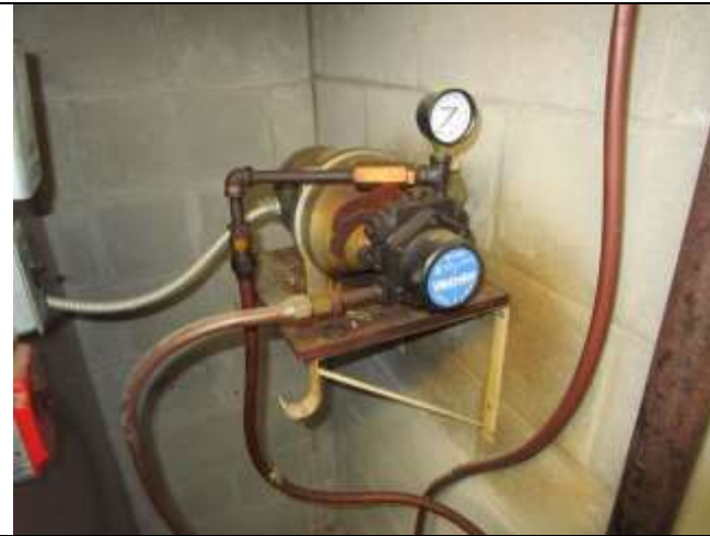
Location: 347 Depot St Jamaica, VT Photo Taken By: Richard Lalancette, P.E. IMG: 195 Description: Fuel transfer pump
