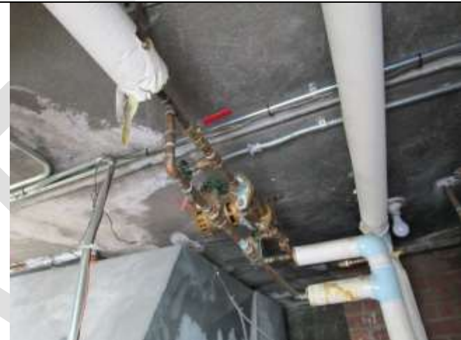
Location: 347 Depot St Jamaica, VT Photo Taken By: Richard Lalancette, P.E. IMG: 193 Description: Circulating pump for circulated hot water system / not operating
