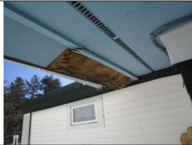
Location: 347 Depot St Jamaica, VT Photo Taken By: Richard Lalancette, P.E. IMG: 143 Description: Soffit repair needed
