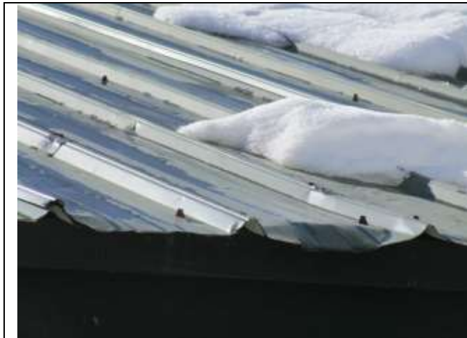
Location: 347 Depot St Jamaica, VT Photo Taken By: Richard Lalancette, P.E. IMG: 176 Description: Damaged roof surface at front entry
