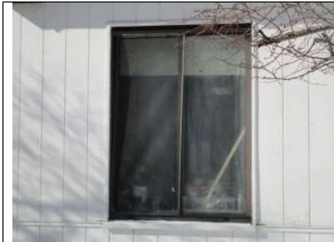
Location: 347 Depot St Jamaica, VT Photo Taken By: Richard Lalancette, P.E. IMG: 139 Description: Fogged thermal pane window
