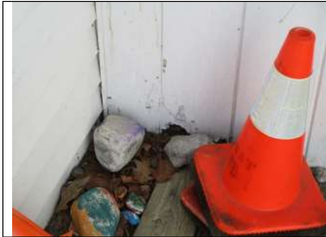
Location: 347 Depot St Jamaica, VT Photo Taken By: Richard Lalancette, P.E. IMG: 142 Description: Rot in lower siding at front of building
