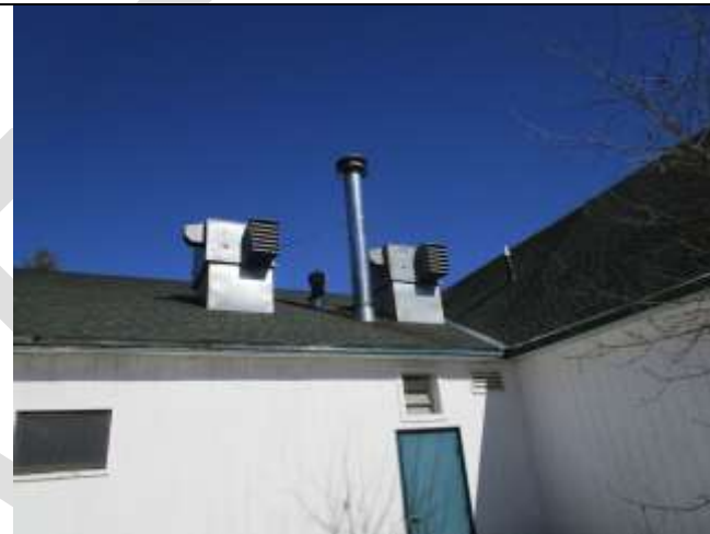
Location: 347 Depot St Jamaica, VT Photo Taken By: Richard Lalancette, P.E. IMG: 181 Description: Metal chimney above roof and heat recovery ventilators
