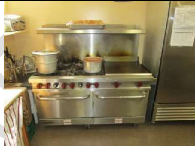
Location: 347 Depot St Jamaica, VT Photo Taken By: Richard Lalancette, P.E. IMG: 201 Description: Kitchen range
