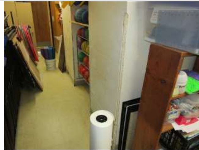
Location: 347 Depot St Jamaica, VT Photo Taken By: Richard Lalancette, P.E. IMG: 203 Description: Storage room off multi- purpose room and damaged sheetrock
