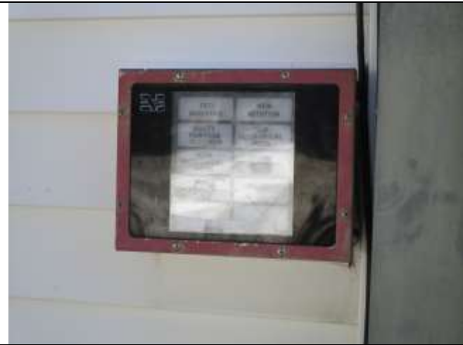
Location: 347 Depot St Jamaica, VT Photo Taken By: Richard Lalancette, P.E. IMG: 151 Description: Remote alarm annunciator
