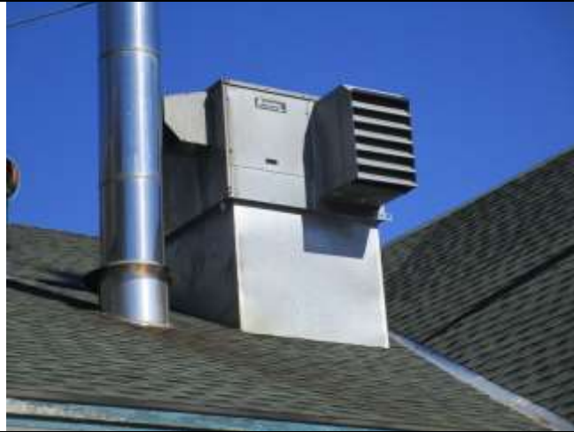
Location: 347 Depot St Jamaica, VT Photo Taken By: Richard Lalancette, P.E. IMG: 183 Description: Heat recovery ventilator
