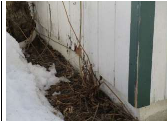
Location: 347 Depot St Jamaica, VT Photo Taken By: Richard Lalancette, P.E. IMG: 160 Description: Rot in lower siding at rear of building
