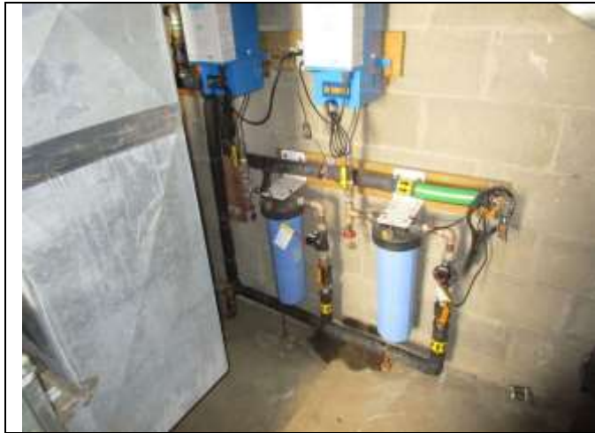
Location: 347 Depot St Jamaica, VT Photo Taken By: Richard Lalancette, P.E. IMG: 190 Description: Sediment filters and ultra violet filters
