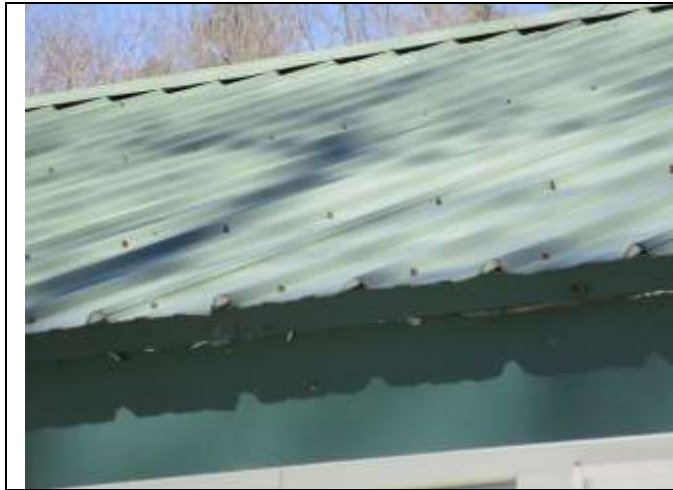
Location: 347 Depot St Jamaica, VT Photo Taken By: Richard Lalancette, P.E. IMG: 178 Description: Raised fasteners at left rear roof surface
