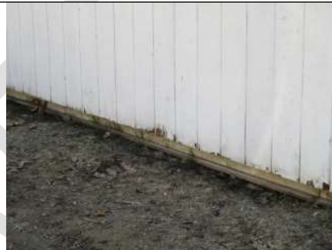
Location: 347 Depot St Jamaica, VT Photo Taken By: Richard Lalancette, P.E. IMG: 165 Description: Rot in lower siding at rear of building
