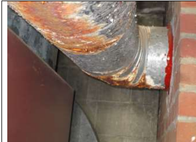
Location: 347 Depot St Jamaica, VT Photo Taken By: Richard Lalancette, P.E. IMG: 192 Description: Deteriorated flue pipe for furnace serving original building
