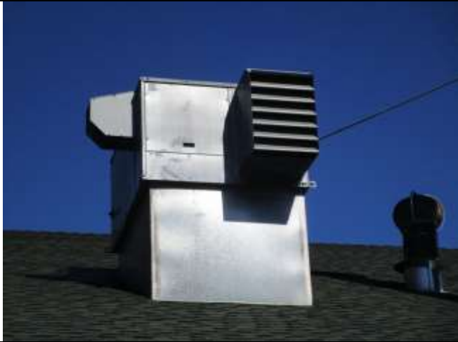
Location: 347 Depot St Jamaica, VT Photo Taken By: Richard Lalancette, P.E. IMG: 182 Description: Heat recovery ventilator
