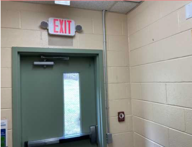
25 - EXIT SIGN WITH LIGHTING PULL STATION.
