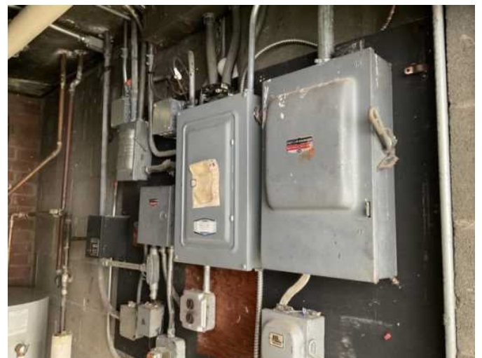
22 - MAIN ELECTRICAL COMPONENTS TO SCHOOL
