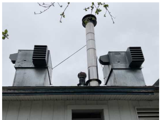
18 - ROOFTOP AIR HANDLER UNIT
