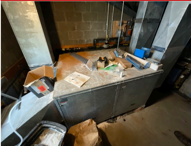
19 - AIR HANDLER UNIT MECHANICAL ROOM
