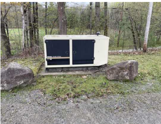
23 - EMERGENCY GENERATOR ALONG DRIVEWAY
