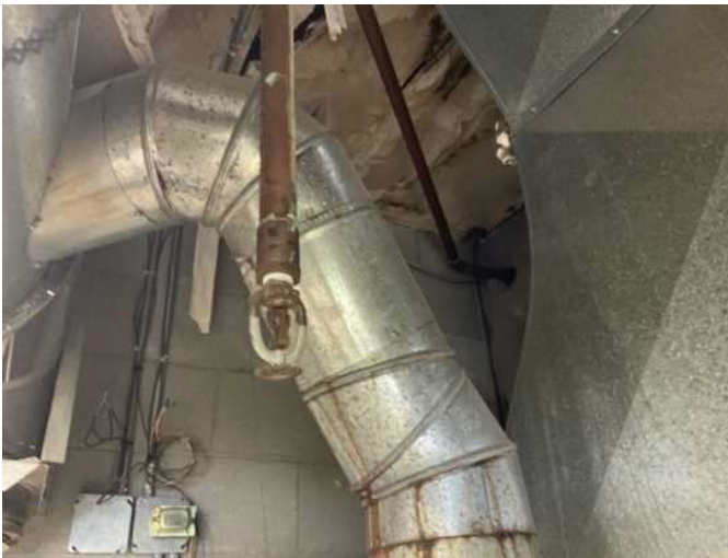
21 - FIRE SUPPRESSION SPRINKLER HEAD
