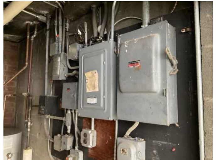
22 - MAIN ELECTRICAL COMPONENTS TO SCHOOL
