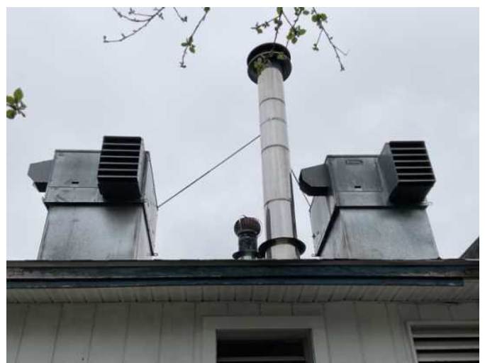
18 - ROOFTOP AIR HANDLER UNIT
