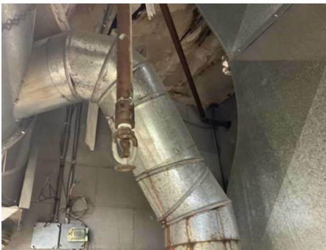
21 - FIRE SUPPRESSION SPRINKLER HEAD
