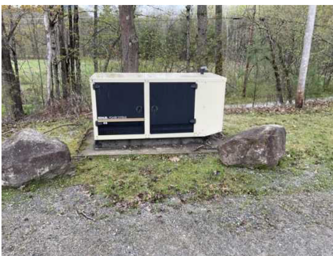
23 - EMERGENCY GENERATOR ALONG DRIVEWAY
