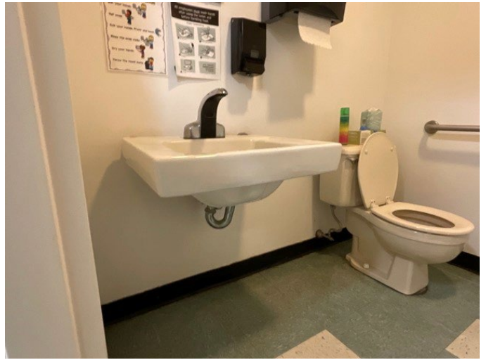
10 - SINK, FAUCET HANDLES
