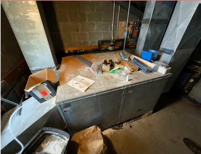
19 - AIR HANDLER UNIT MECHANICAL ROOM
